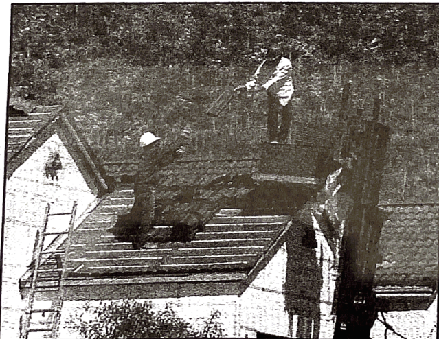
Construction workers load tile onto the roof of a home at Sabino Springs.
